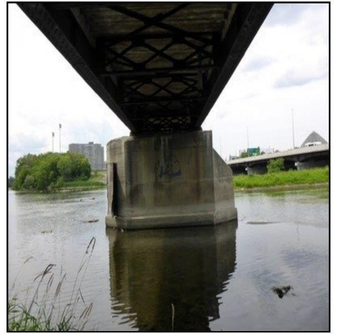
The bridge's piers remain visible when the Rideau is low, and are its last remnants.
